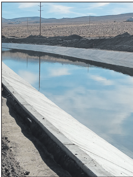
Portion of lined area of Truckee-Canal taken in December. Photo by John Clodius.
