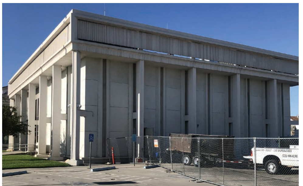
The old jail is being removed from the ground floor of the District Court building, forcing two county departments to relocate while work is done. Photo by Anne McMillin.
