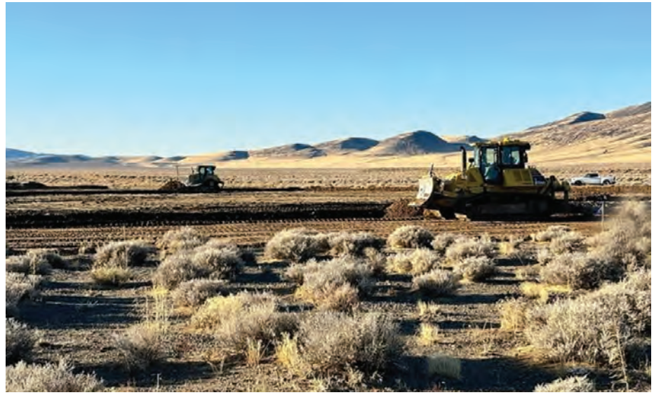
NV Energy’s 400-megawatt solar field project. Photo courtesy of NV Energy.
