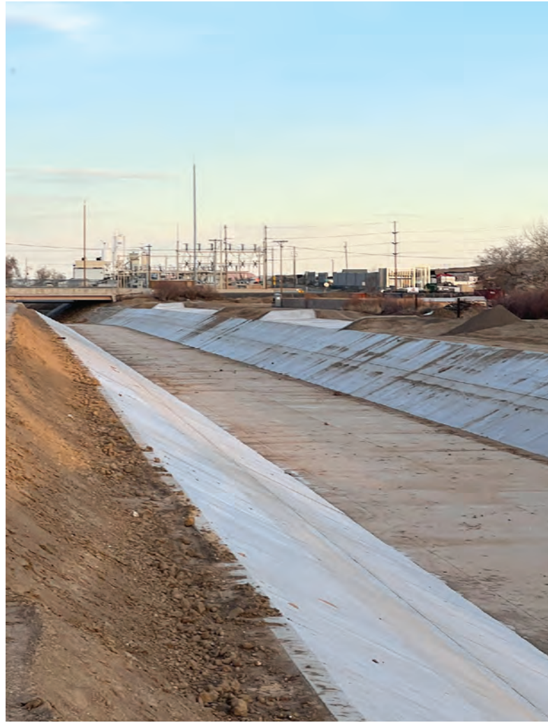
Fernley's Truckee Canal upon installation of new concrete lining. Photo by Leanna Lehman.
