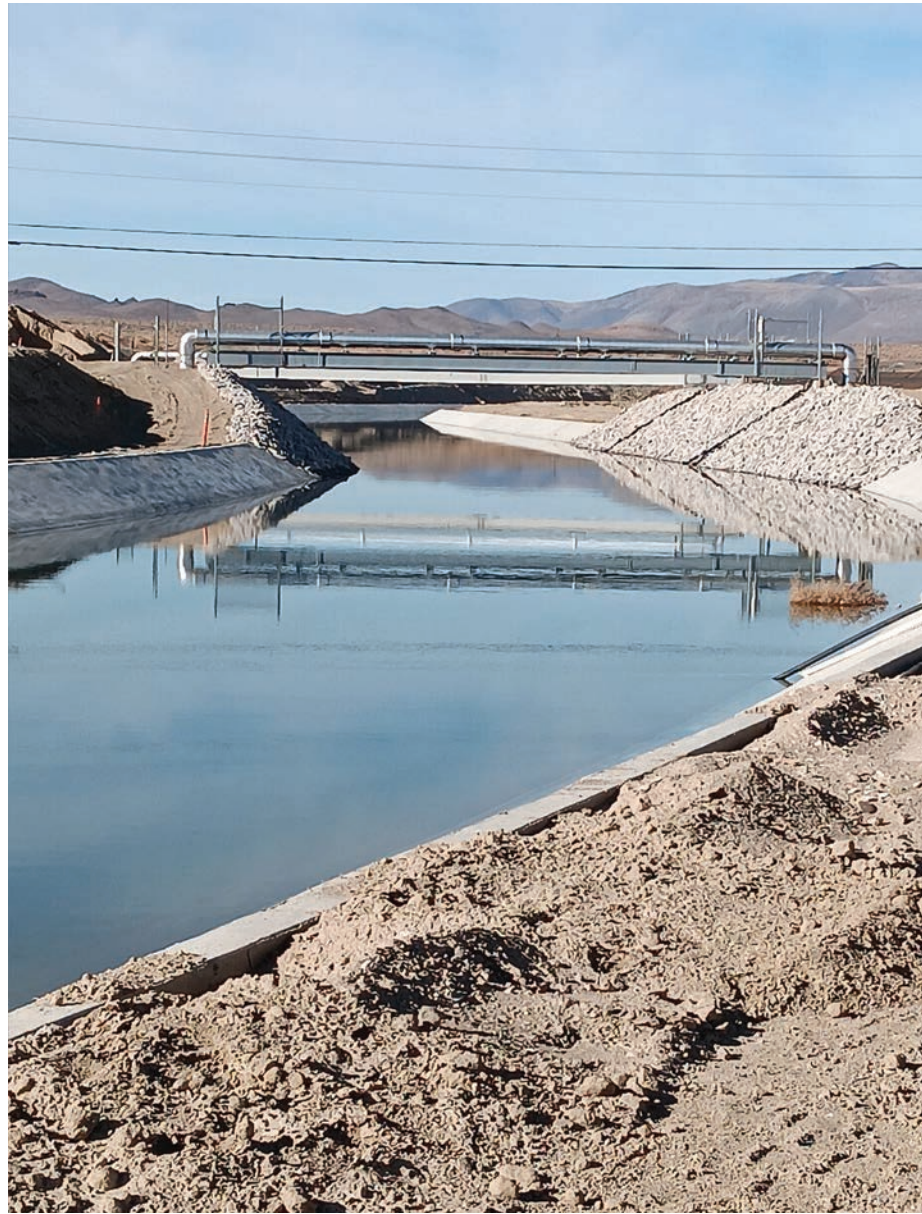
Truckee Canal shortly after construction completed on 3.1 mile stretch of concrete lining, December 5, 2023. Photo by John Clodius.
